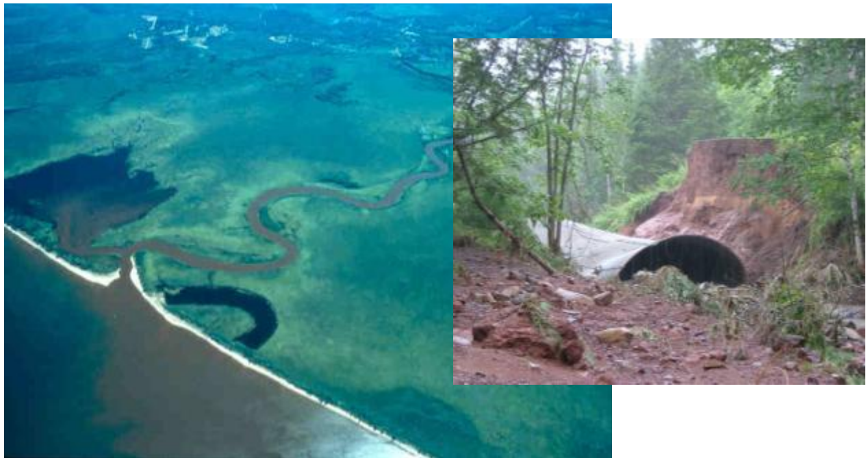
Figure 2. Mouth of the Bad River, and a destroyed culvert after a blowout event.
